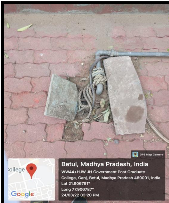
Behind Control Room
